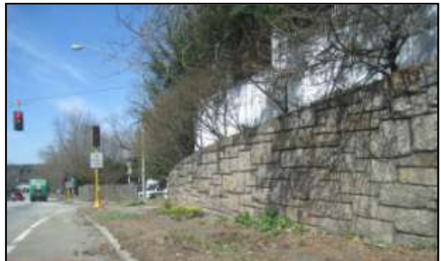
Poorly maintained sidewalk in Wellesley
