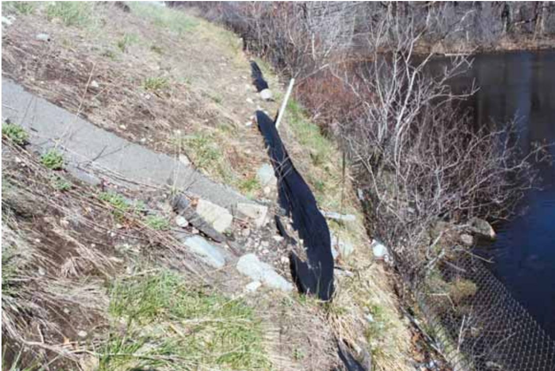
Figure 4-4 Unstable Turnpike Embankment on Middle Pond
