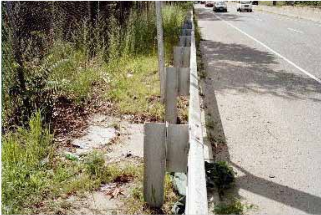
Figure 4-3 Stormwater overtops curb onto embankment, Route 9 at South Pond
