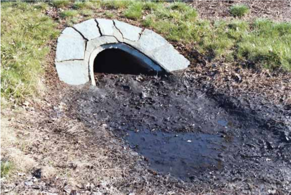
Figure 4-6 Clogged Drainage Outlet at Natick Service Plaza
