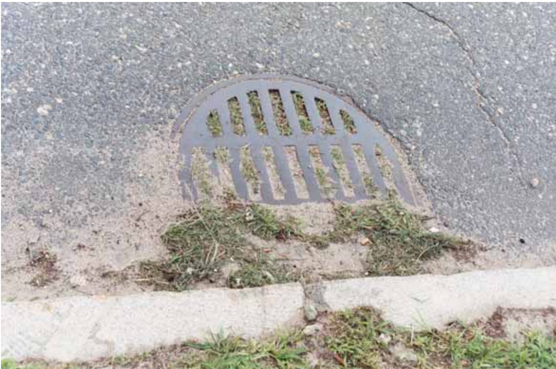
Figure 4-2 Clogged Catch Basins, Route 9 at South Pond
