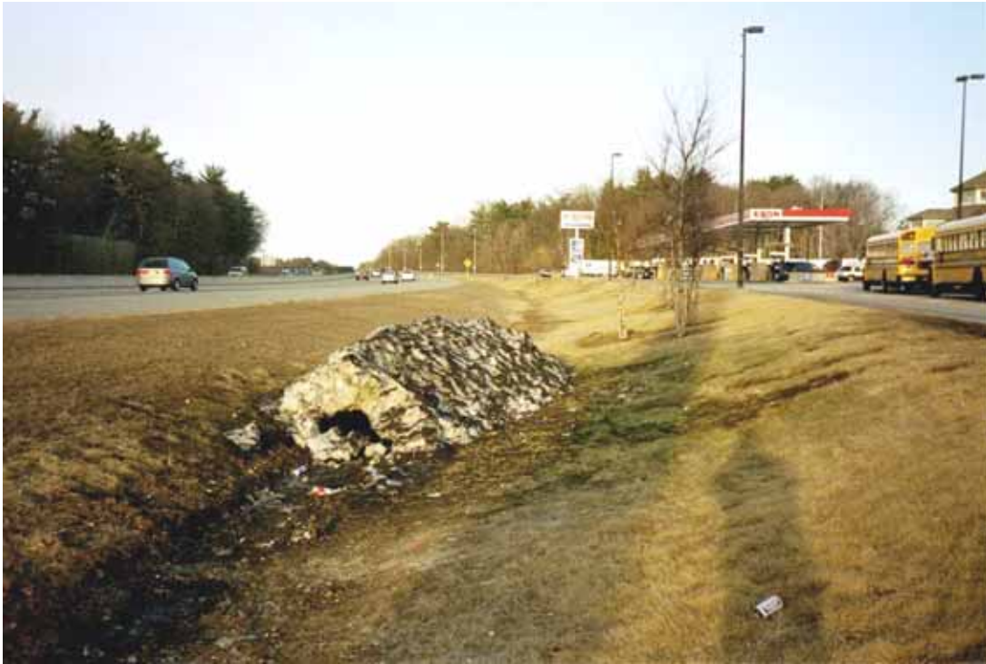
Figure 4-8 Sediment laden snow pile in drainage ditch, Natick Service Plaza
