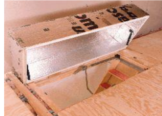
An insulating dome installed above attic stairs prevents cold air from drifting down through the hatch
