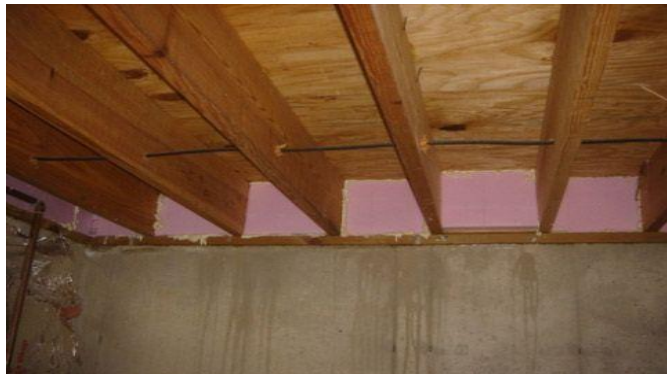
Rigid insulation installed along the rim joist prevents cold air from being pulled into the basement
