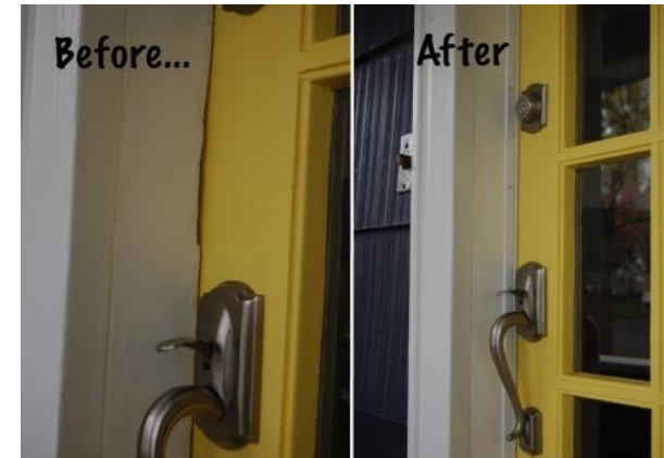
Weather-stripping prevents drafts around doors
