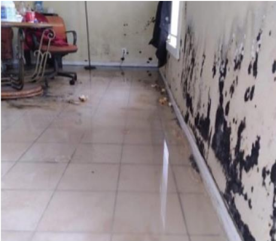
Mold in occupied rental housing in Mississippi
