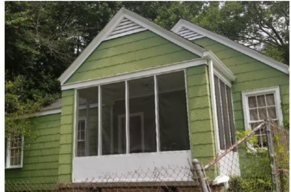
Housing unit repaired through the Lead Safe Jackson Housing Program, where lead paint hazards were identified in the screen porch and child's outdoor play area.
