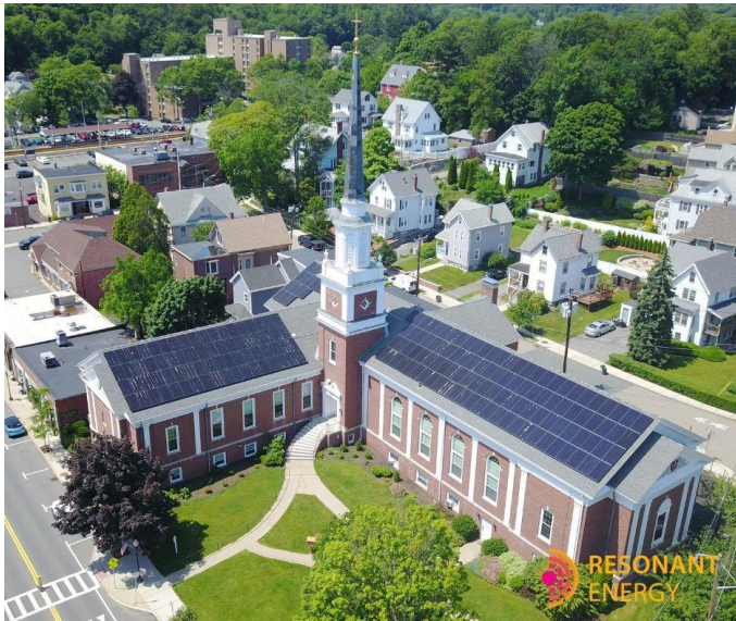
A solar PV system installed at the Melrose Highlands Church. Source: City of Melrose .
