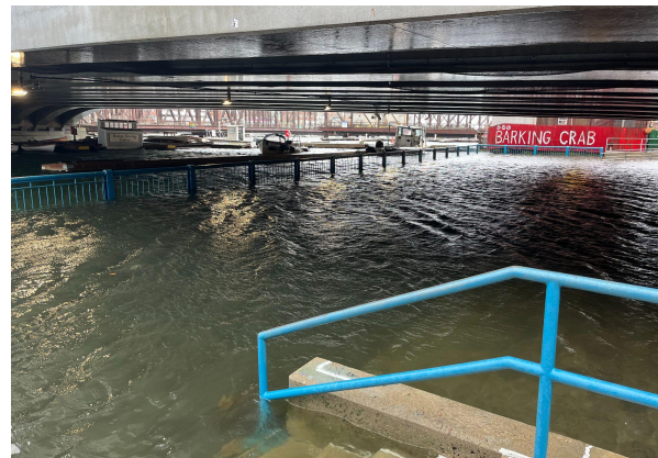
Flooding beneath the Evelyn Moakley Bridge in South Boston's Fort Point Channel (Source: Alison Brizius, December 2022)
